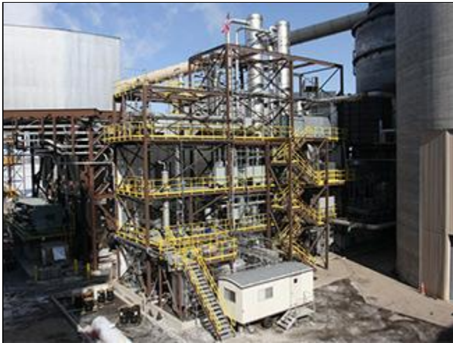
Alstom and the Electric Power Research Institute have opened this plant in Wisconsin to test the use of chilled ammonia to capture CO2 from power plant emissions. Photo courtesy of Electric Power Research Institute.
